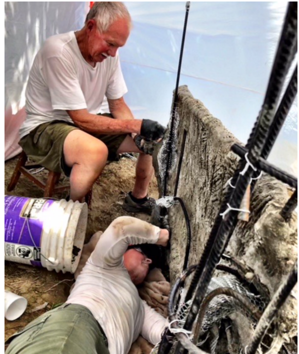
Gerry Crawford and Mary Jo working on the back of the bench
